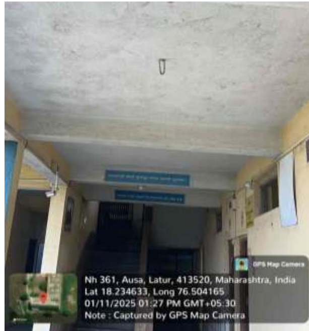
CCTV Camera in veranda
