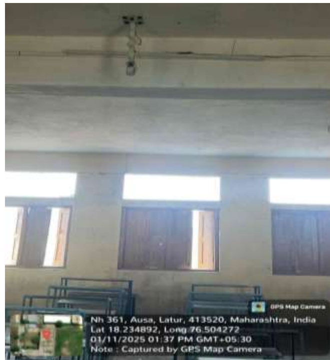
CCTV In Class Room 213
