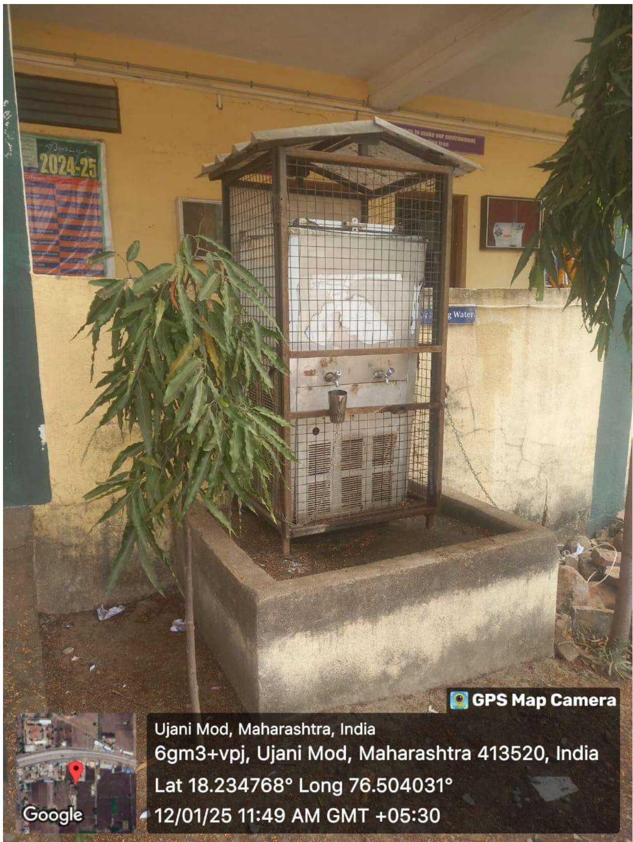
DRINKING WATER FACILITY
