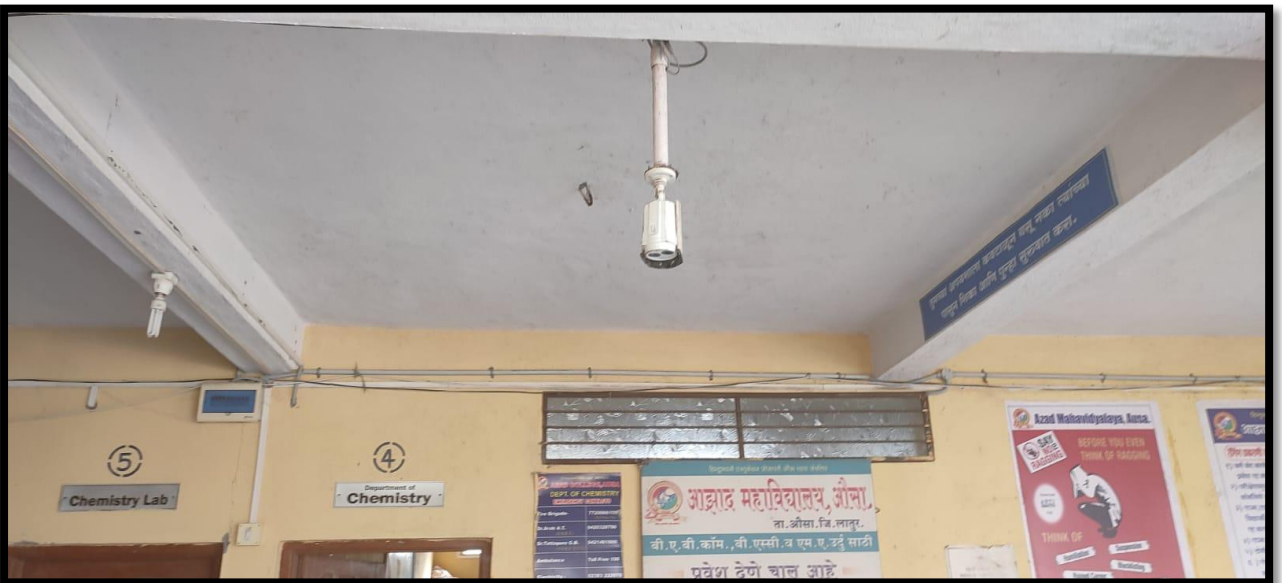
CCTV camera in Varanda at First Ground Floor nearby chemistry Dept.
